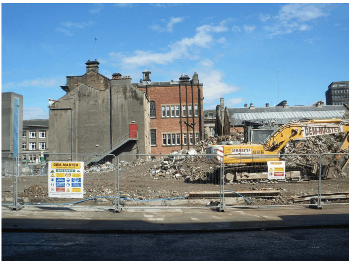
Glasgow Meeting House, with Scottish Opera behind, HS both dwarfed by the bulldozer.
